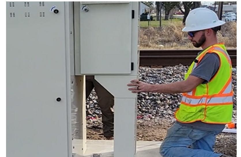
A hydrogen supplier installs a new hydrogen-powered fuel cell at a Union Pacific crossing in Louisiana.
