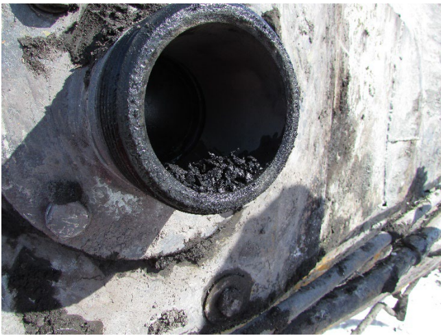
5(f) Bottom outlet valve gasket thermally damaged.
